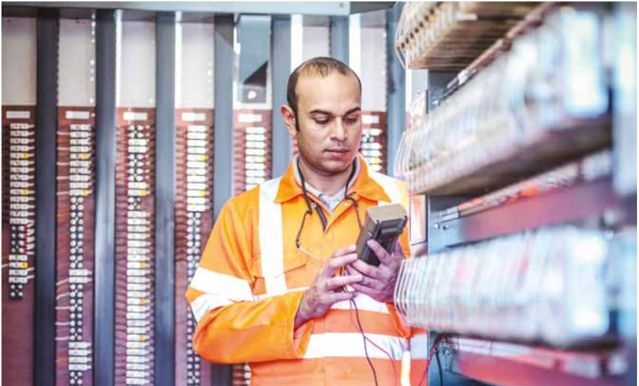
Image courtesy of Schneider Electric (Hong Kong) Limited
