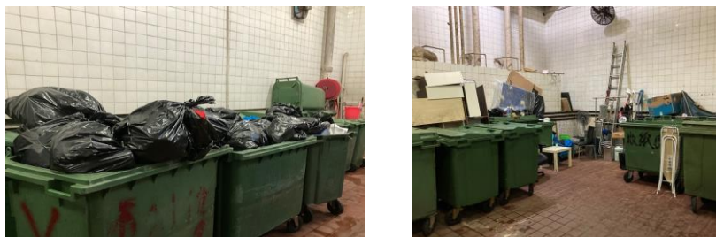
A central refuse storage and materials recovery room located at the parking lot of the housing estate.
