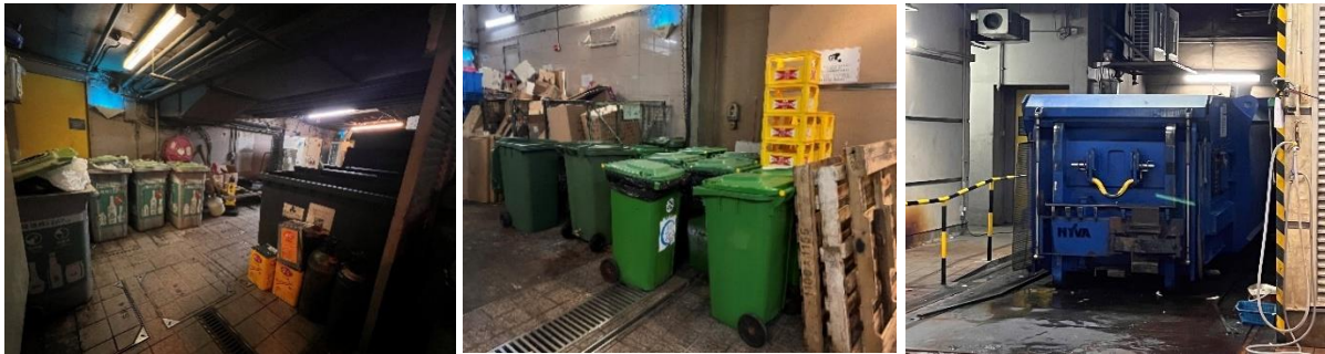
A central refuse collection and storage point at a hotel basement, with collection bins for different waste streams (left and middle) and a waste compactor (right) in place.
