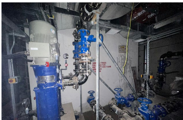
Rainwater recycling system
