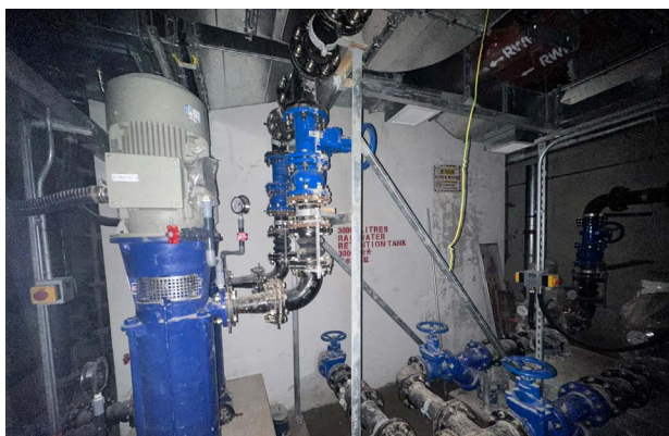
Rainwater recycling system
